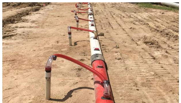
Vertical well-point system
