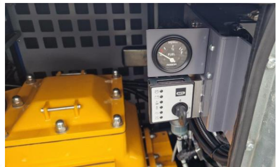
Engine controller inside canopy
